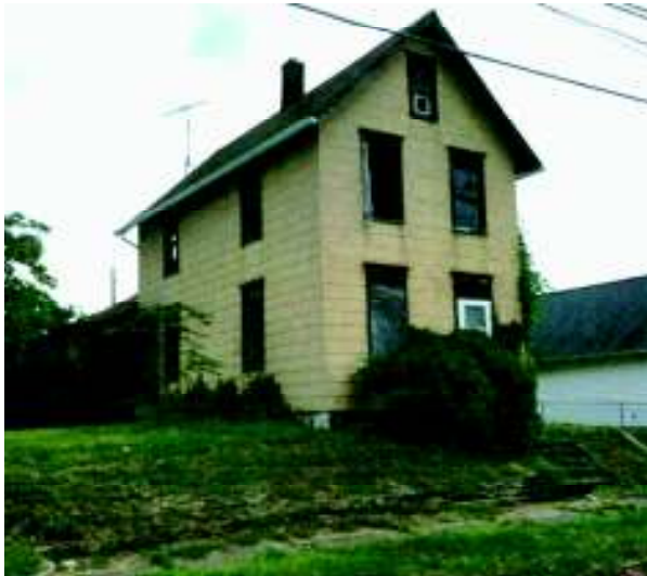
Blighted property on 3rd Street SE, Canton, OH - to be demolished with the use of NIP funding
